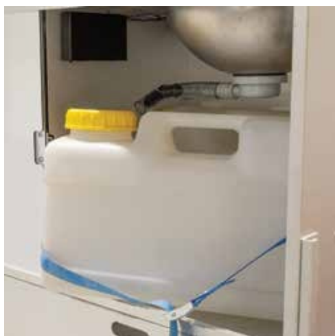
Picture 14. Drainage canister disconnected.
