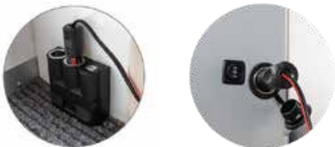
Picture 12. Cable connection between the trailer and the kitchen.
