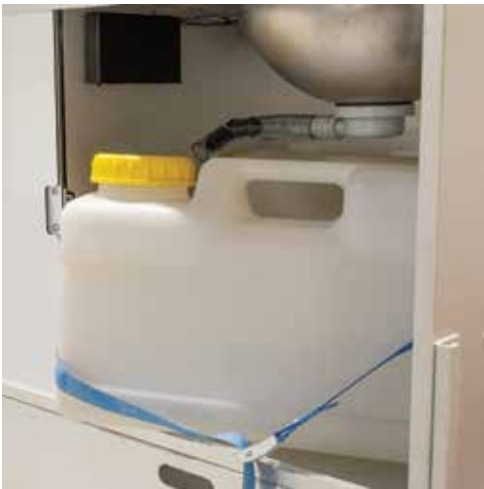
Picture 14. Drainage canister disconnected.
